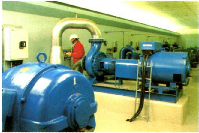
The effects of water hammer in the pipes is eliminated by the slow start and stop of the pumps.
